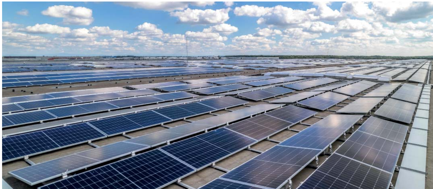
VGP Park Timisoara, solar panels
