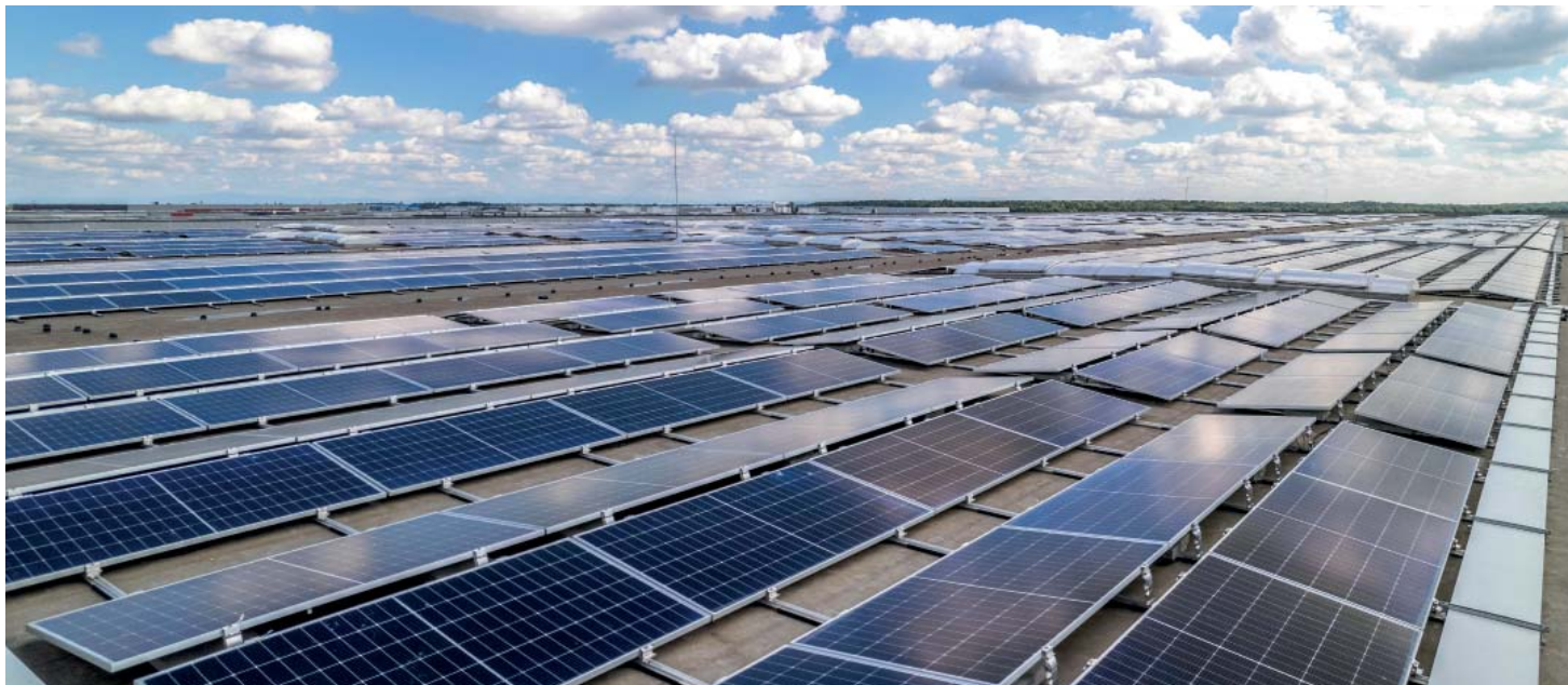
VGP Park Timisoara, solar panels
