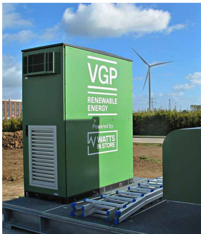
Battery Energy Storage System in VGP Park Nijmegen, The Netherlands
