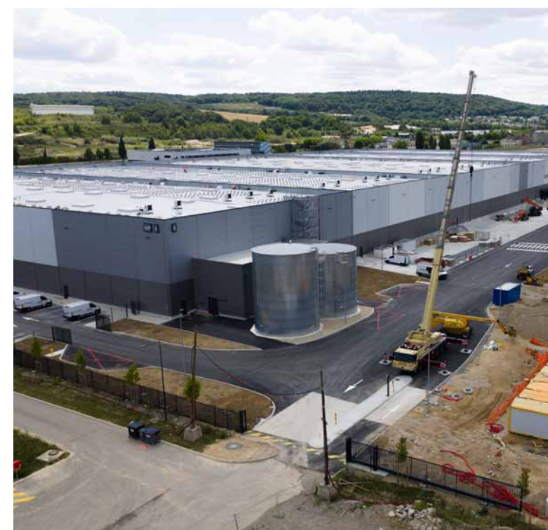
VGP Park Rouen combines brownfield regeneration, low-carbon materials, and high waste recovery to keep resources in use and reduce environmental impact
